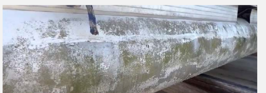
UNPROTECTED TRITON SHOWING CORROSION
